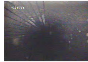
Down View - showing patches of moderately clogged SS Screen at 156.5 mbgs at 87.9 mbgs
